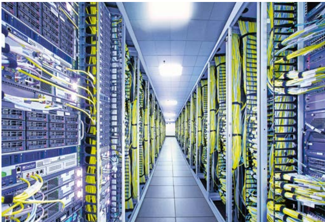
Demanding data center application
